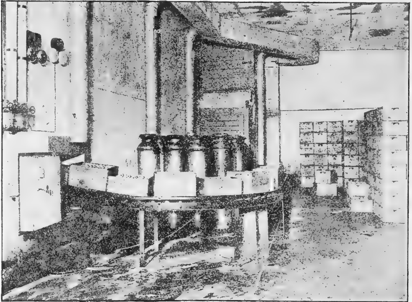
FIG. 14.—Milk-storage room with indirect system of cooling. Note flues through which the cold air is fanned into the room, also system of conveying the milk into the room from the bottling room.
